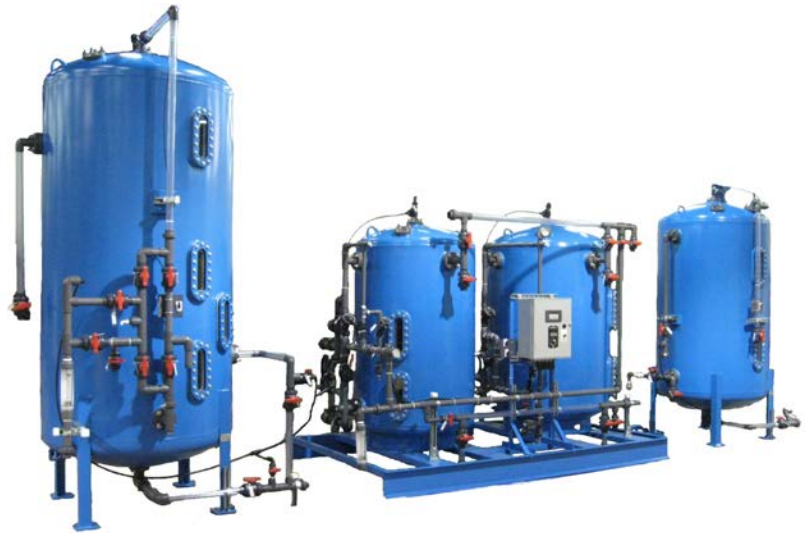
60 ft 3 Regeneration Plant
